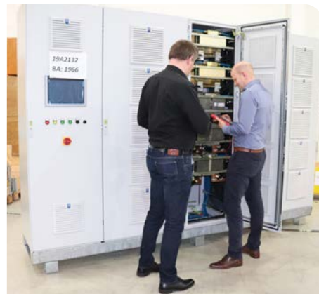
Inspection of water-cooled throttles of one out of four 3 MVA frequency converters of the test station
