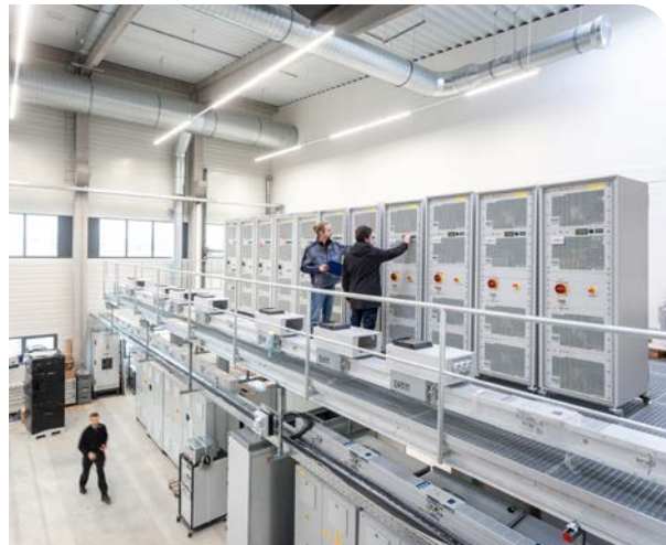
Multi-megawatt laboratory at the centre for power electronics and sustainable grids
