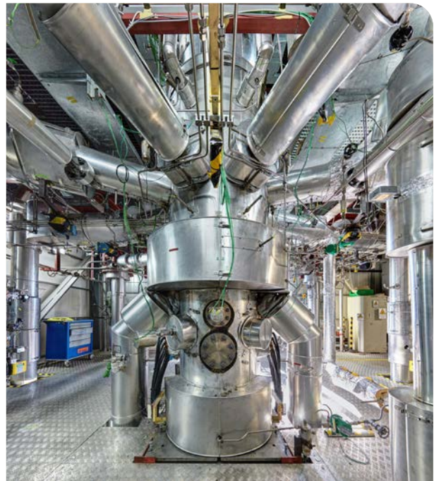
Reactor pressure vessel of the primary coolant loop (PKL) test facility with main coolant pipes of Framatome GmbH
