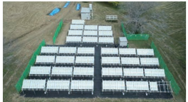
Photocatalyst water-splitting panels with an area of 100 m 2
