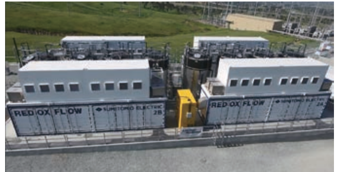
Microgrid operation with a large-scale battery system on an in-service distribution network (Demonstration in the U.S. state of California)
