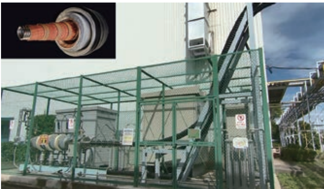
Demonstration of a three-phase coaxial superconducting cable
