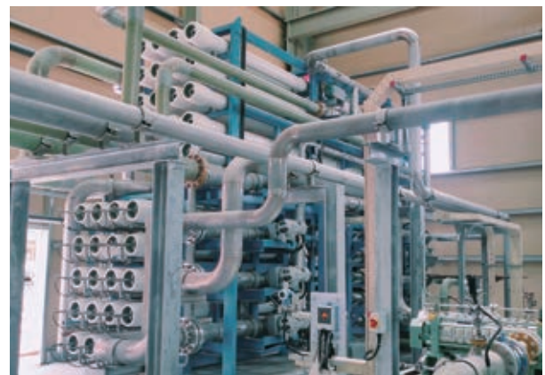
Energy-efficient seawater desalination plant (Saudi Arabia)
